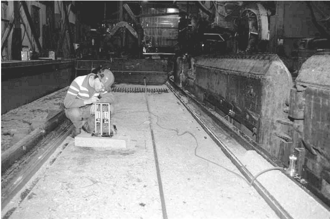
Figure 17. Using a precision water hose level to measure the elevations of the V- and flat rails. The reading is being taken at the base unit, while the measurement vial is on the flat rail in the right side of the picture.
